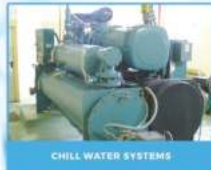
CHILL WATER SYSTEMS
